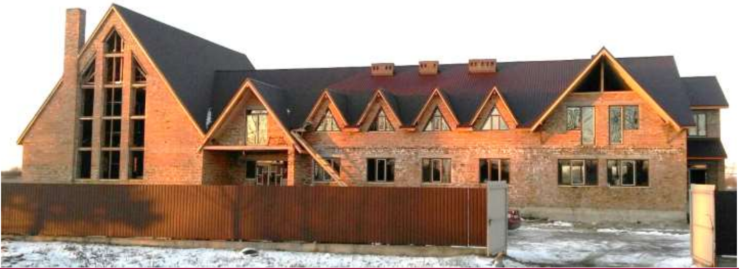
Photo: The roof is finished; exterior doors installed; all windows except the large windows installed!!
